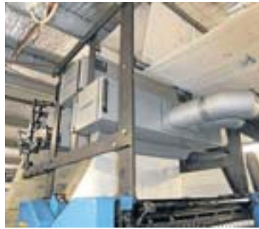
Far left, the Bairnsdale crew and suppliers show the results of their UV installation, and (left) the Prime UV unit in place on the press.
